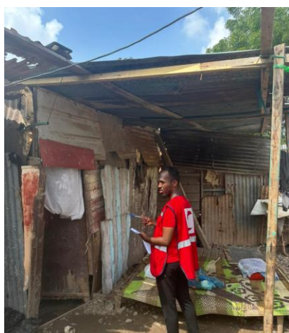
Rusted and weak roofing, Nov 2023 @DRCS Photo Credit: - DRCS
